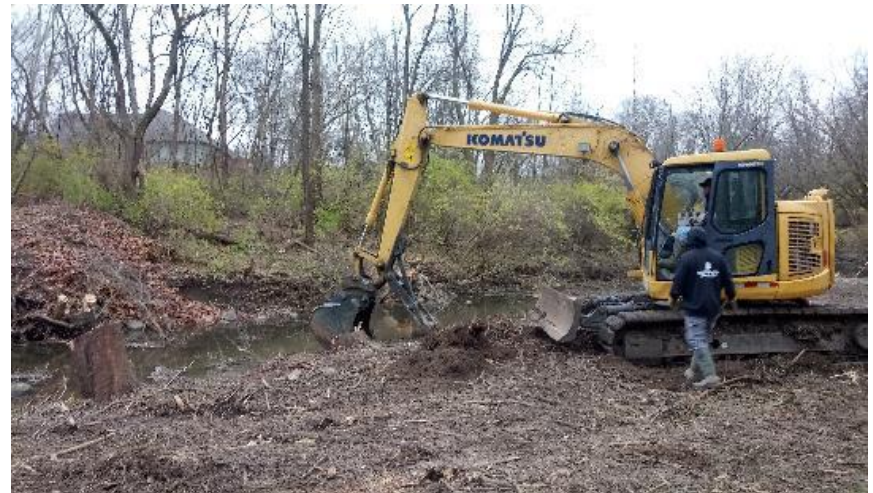
Removing a tree stump while clearing, west of the creek at STA: 28+00
