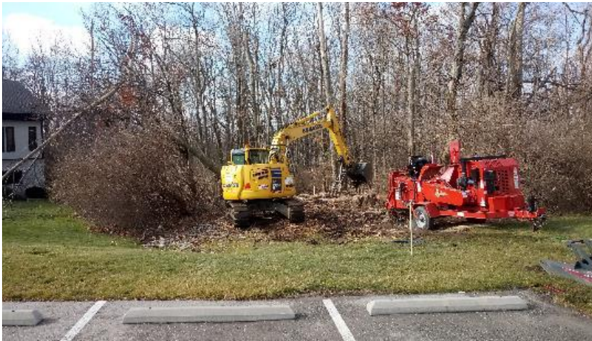
Start of clearing operations at the end of Hornet Avenue, next to Skillman building.
