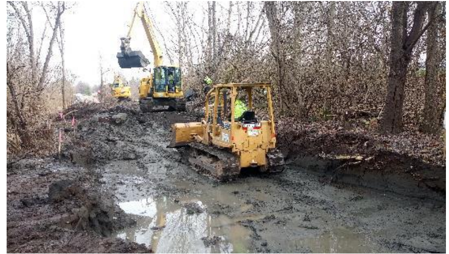
Dozer pushing sloppy material to an excavator that loaded it out on trucks.
