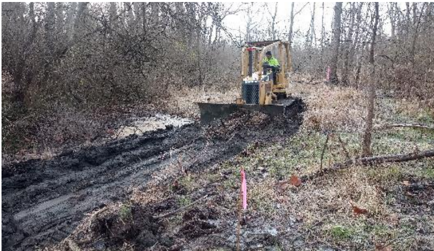
Dozer pushing the soft, muddy surface grade to prepare for subgrade treatment.
