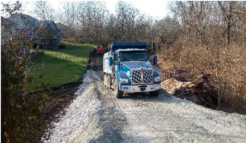
Truck backing down the stone ramp built for construction access, east of Lick creek.
