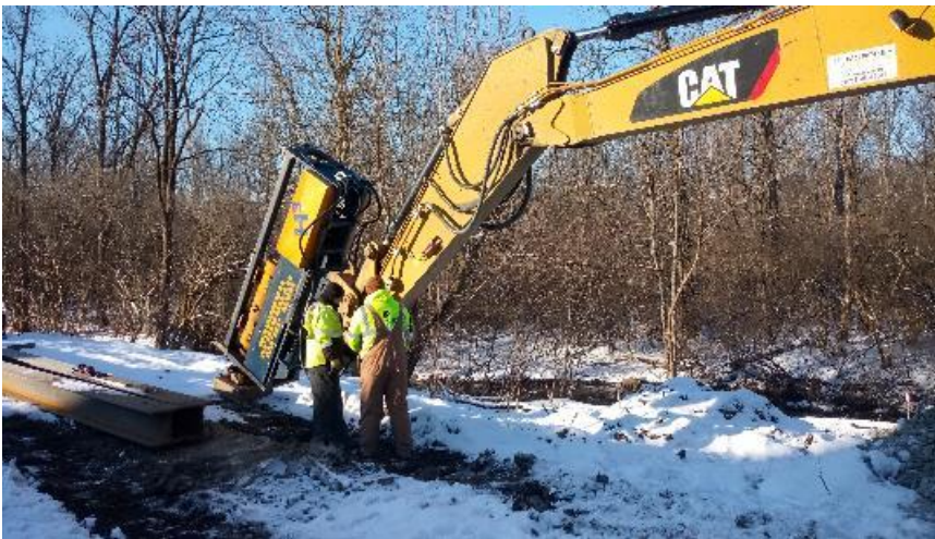
Morphey adjusting the hammer on the excavator before moving it to Bridge #2.
