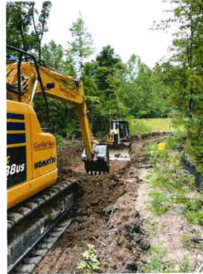
Undercut West of bridge 3
