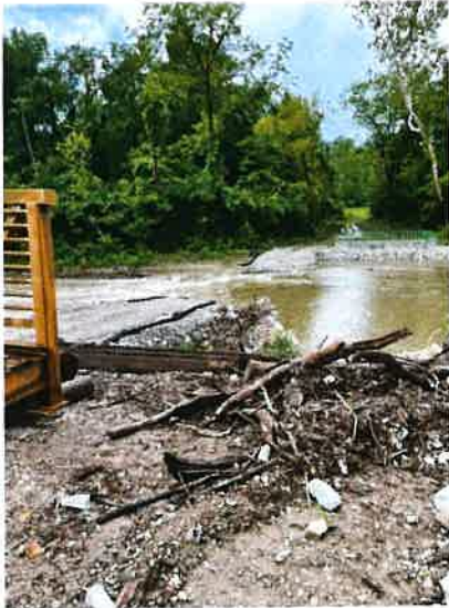
Flooding at Bridge 3
