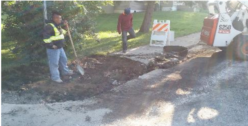
Sidewalk tear out on northeast corner of 12th Avenue and Alton Street.
