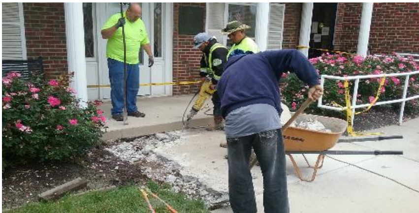
Demo work on sidewalk in front of City Hall for new ramp approach.
