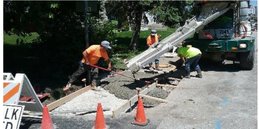
Pouring concrete curb ramp, northeast corner of 12th Avenue and Alton Street.
