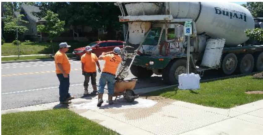
Pouring concrete in wheelbarrow to transport to location of new City Hall ramp.
