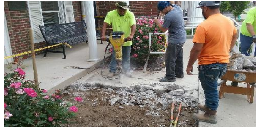
Demo work on sidewalk in front of City Hall for new ramp approach.
