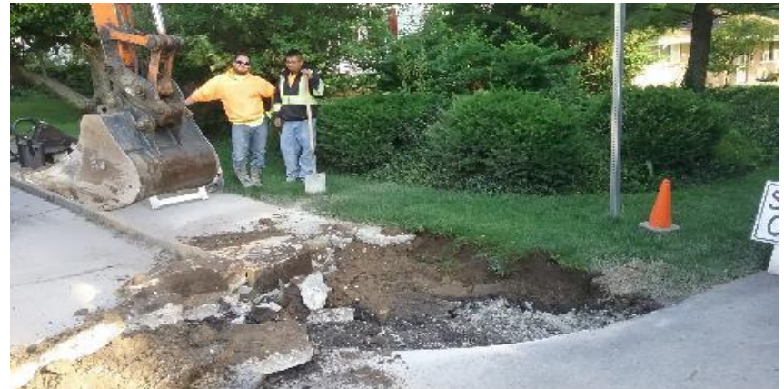
Sidewalk tear out on northwest corner of 12th Avenue and Alton Street.
