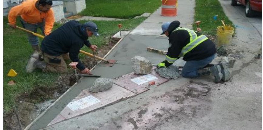
Finishing ADA ramp on southeast corner of 7th Avenue and Buffalo Street.
