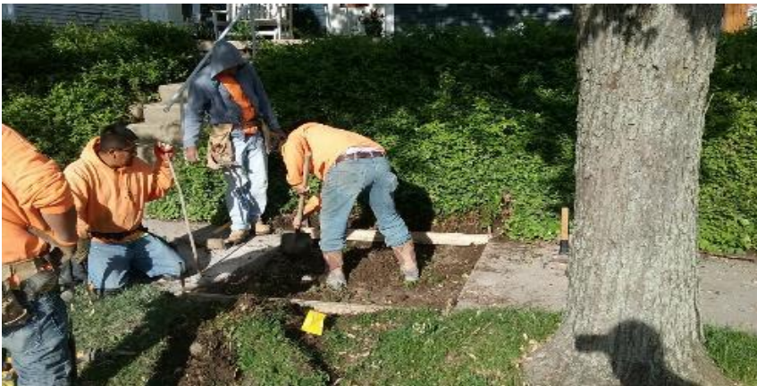
Forming sidewalk, west side of 9th Ave, between Albany St. and the alley.
