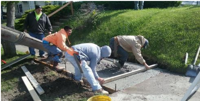
Pouring concrete sidewalk on 9th Avenue between Albany St. and the alley.
