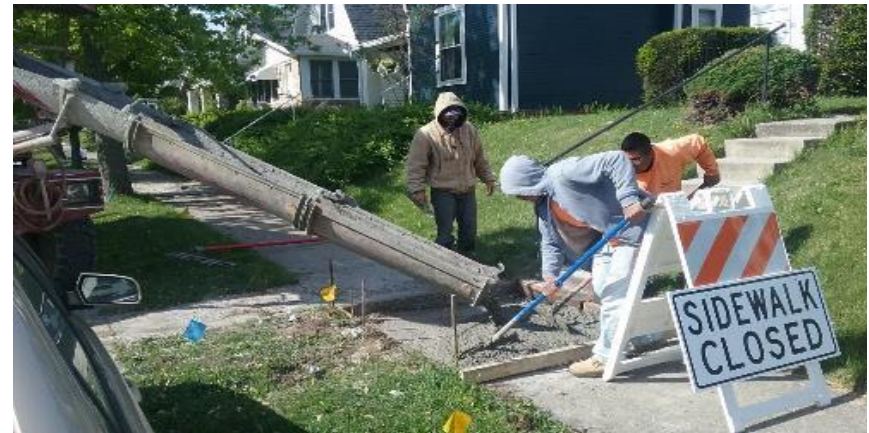
Pouring concrete sidewalk on 9th Avenue between Albany St. and the alley.
