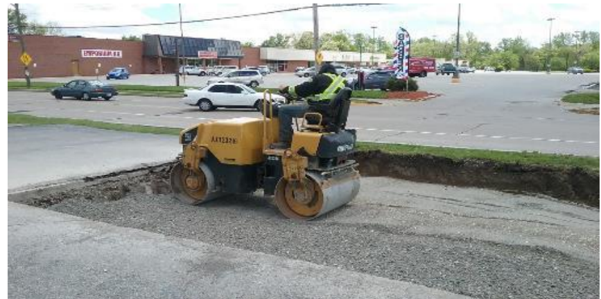
Compacting subgrade for the new lowered grade of the Henthorn parking lot.
