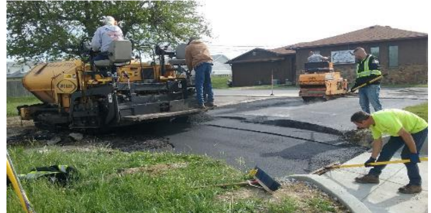
Placing surface asphalt at the Henthorn lot up to the concrete approach.
