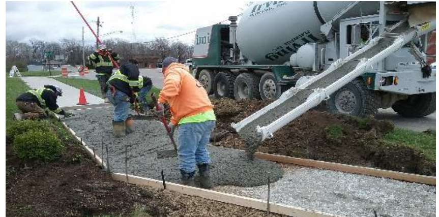
Pouring sidewalk transition from existing to ADA ramp east of Schaff St.
