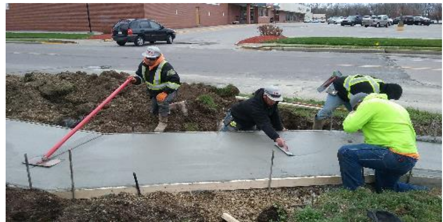
Finishing sidewalk transition from existing to ADA ramp east of Schaff St.
