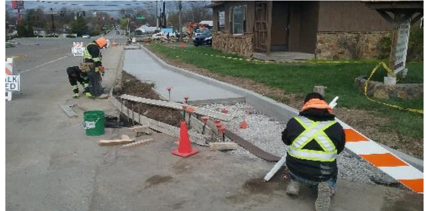
Forming curb and ADA curb ramp on the west side of Schaff Street.
