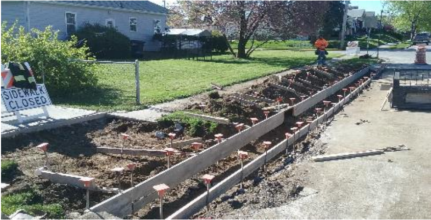
Forming approach at 166 N. 9th and curb, just north of Albany St.
