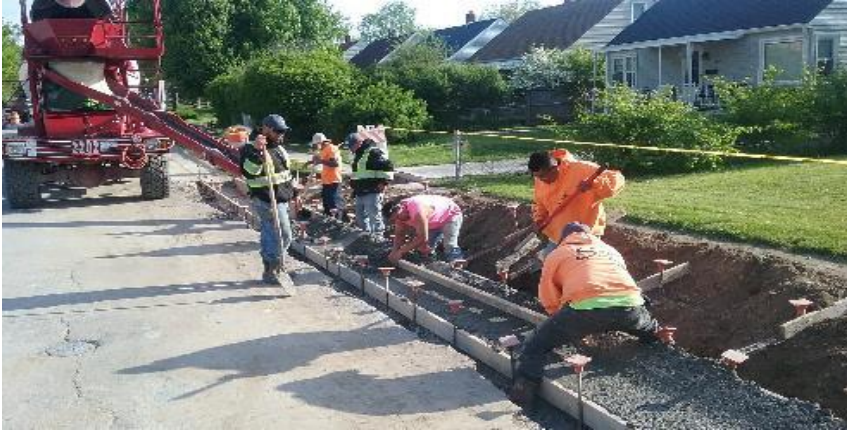
Pouring curb and gutter on the east side of N. 9th Avenue.
