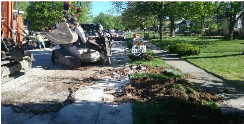
Hammering out existing curb to be replaced east of N. 9th Avenue.
