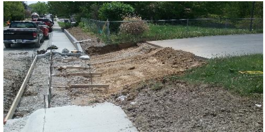
Curb and sidewalk removed at 174 N. 9th Ave for lowering of approach.
