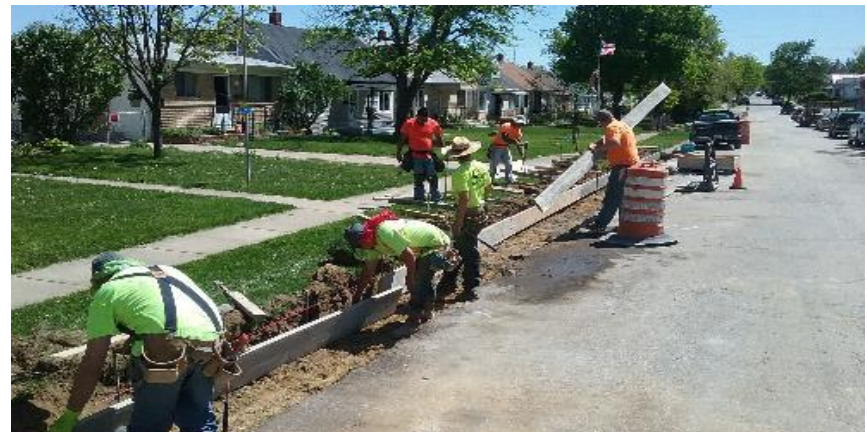
Forming curb and gutter on the east side of N. 9th Avenue.
