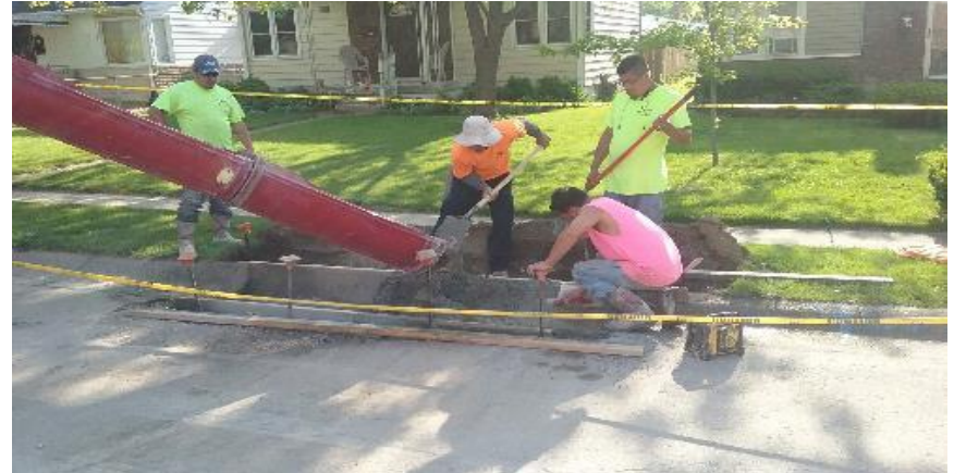
Pouring curb and gutter on the east side of N. 9th Avenue.
