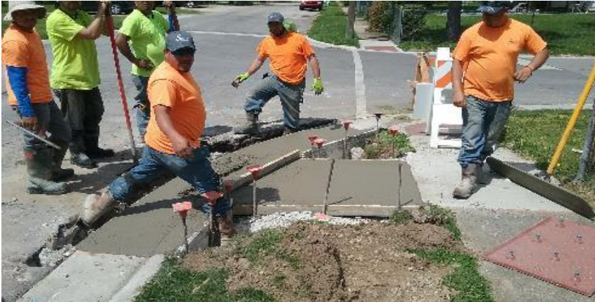
Finishing ADA curb ramp on southeast corner of 9th Ave. and Buffalo St.
