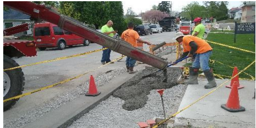
Pouring concrete sidewalk in front of the Wilmar Apartments, north 9th Ave.
