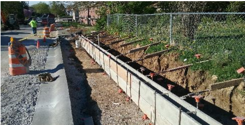
Modified curb forms on the backside of the sidewalk at 174 N. 9th Avenue.
