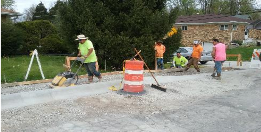
Compacting and prepping for sidewalk, west of 9th Ave, south of Buffalo St.
