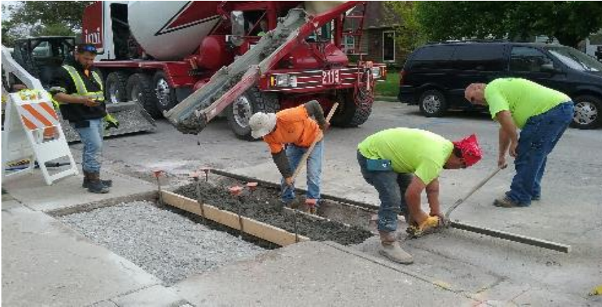
Placing concrete for curb and gutter in front of 166 N. 9th Avenue.
