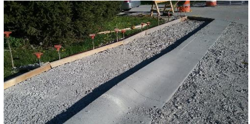
Sidewalk formed on the west side of 9th Avenue leading up to Buffalo St.
