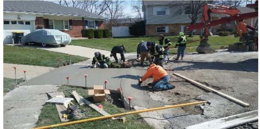
Finishing the curb and driveway approach in the Cul-de-saq at 502 St. John's Ct.
