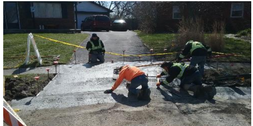
Finishing the curb and driveway approach in the Cul-de-saq at 417 St. John's Ct.
