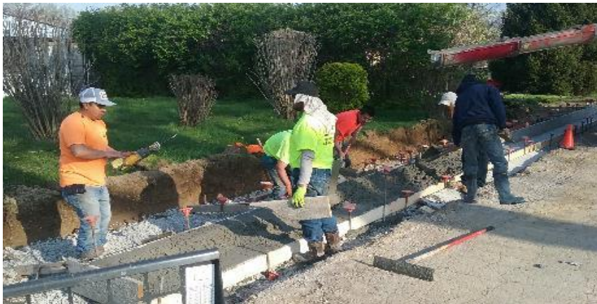
Pouring concrete curb and gutter on westside of 9th Ave, south of Buffalo St.
