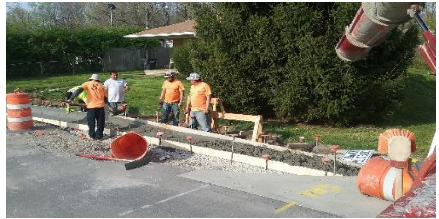
Finishing concrete curb and gutter on westside of 9th Ave, south of Buffalo St.
