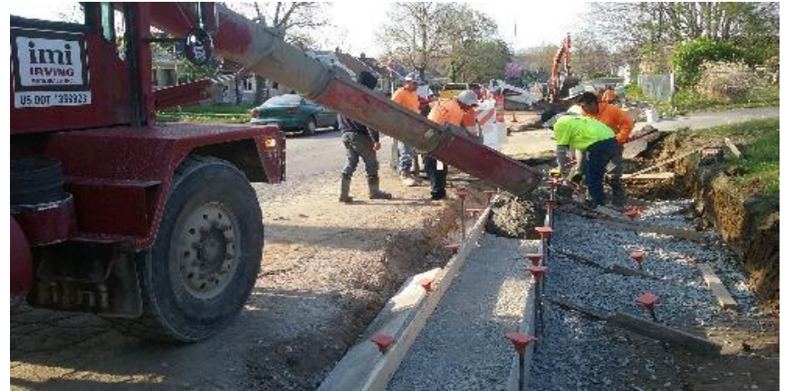
Pouring concrete curb and gutter on westside of 9th Ave, south of Buffalo St.
